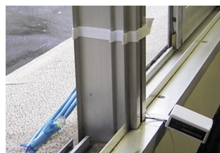
Fig. 9. Example of the fixture of the developed flat cable on the window frame.
