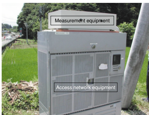
Fig. 1. Access network equipment.
