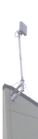
Fig. 8. Pole mounted under eaves.
