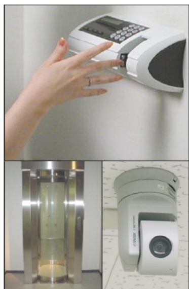
Fig. 3. Security at NTT West Osaka Data Center. Top: Biometric personal identification system; bottom left: system for preventing entry by multiple persons; bottom right: blind-spot-free surveillance camera.
