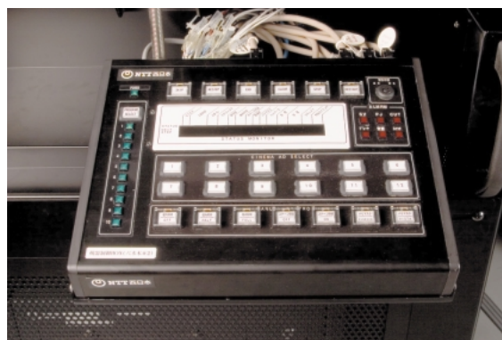
Fig. 2. Theater control box.
