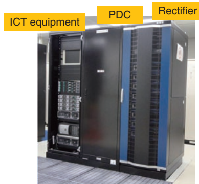
PDC: power distribution cabinet
