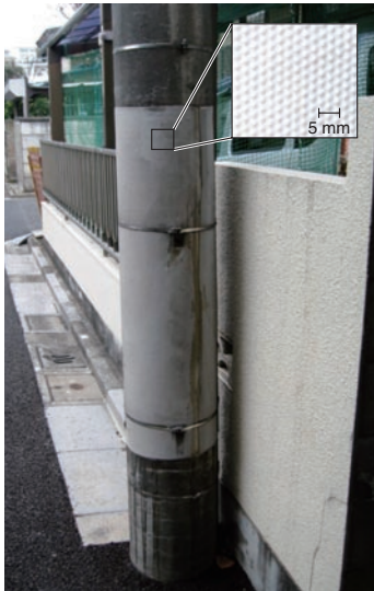
Fig. 1. Bill-posting prevention sheet on a concrete pole.
