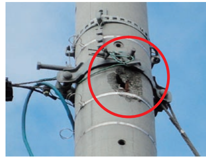
Fig. 3. Damage to CP (detachment of concrete from surface of CP).
