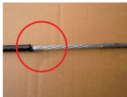
Fig. 1. Damage to messenger wire.
