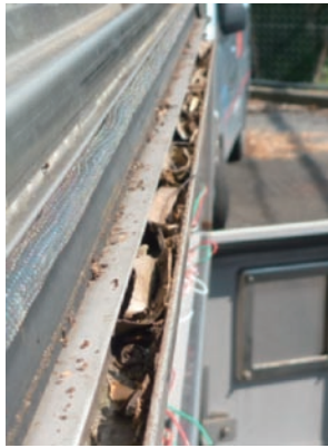
Fig. 4. Clogged drainage duct.
