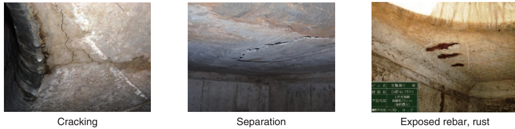
Fig. 3. Types of manhole degradation.
