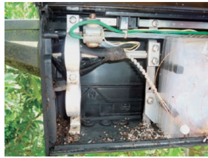
Fig. 5. Closure that has been penetrated by ants.
