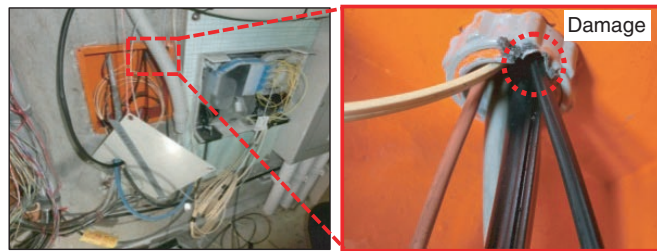
Fig. 6. On-site conditions (MDF room).
