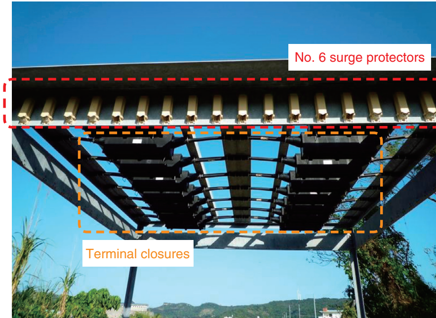
Photo 1. Facility using humidity-controlling polymer (foreground: No. 6 surge protectors; background: terminal closures).
