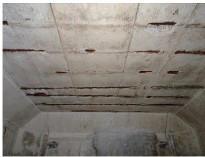
Fig. 4. Degradation of upper floor plate (exposed reinforcing bars).
