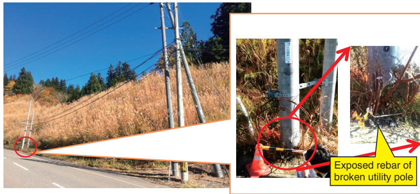
Fig. 1. Site of snow damage and state of broken concrete utility pole.
