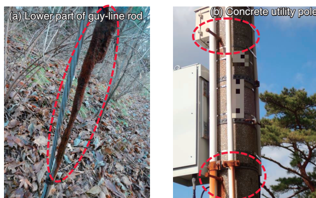
Fig. 3. Examples of sulfur damage to outdoor facilities.
