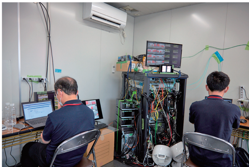
Fig. 4. NTT network equipment that provided ultra-low-latency communication technology.
