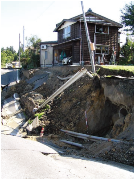
Fig. 1. Exposed conduits in a collapsed road.
