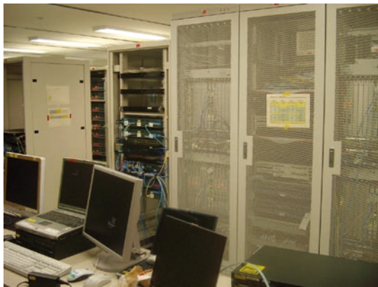
Photo 1. NGN testing area. Researchers perform comprehensive testing by simulating an actual network environment to enable stable operation of NGN field trials and to facilitate system deployment. The racks hold many servers of various types.
