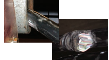
(3) Damage at conduit separation
