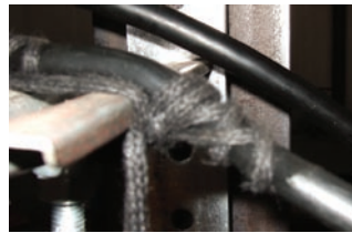
(2) Damage at metal fixture
