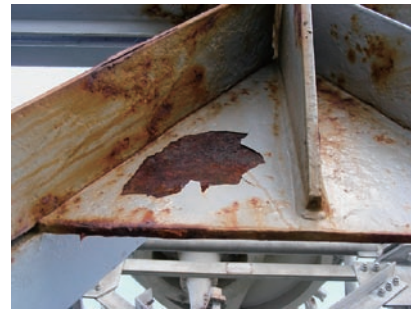
Fig. 4. Example of corrosion in steel materials (red rust).
