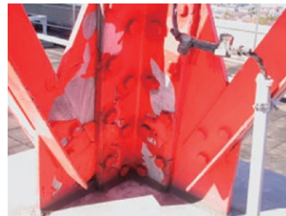
Fig. 6. Example of peeling.
