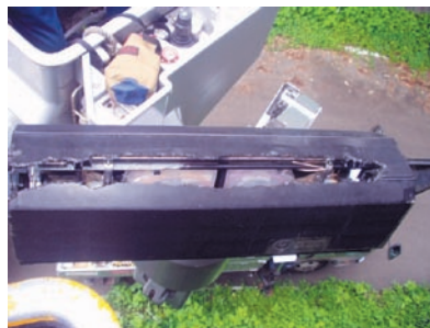
Fig. 4. Damage to an FFA closure (by a squirrel).
