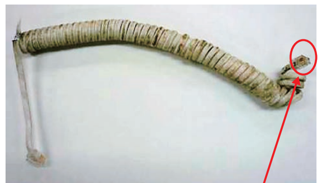
Broken modular plug
