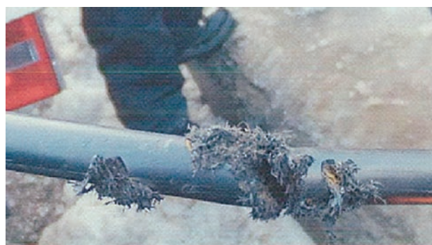
Fig. 2. Damaged optical cable with open cut.
