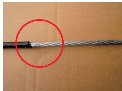
Fig. 1. Damage to messenger wire.
