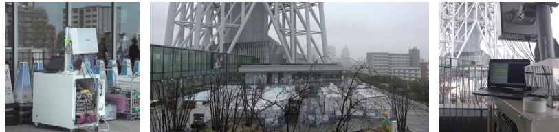
Construction of 5G communication environment at Sky Arena on 4th floor of Tokyo Skytree Town
