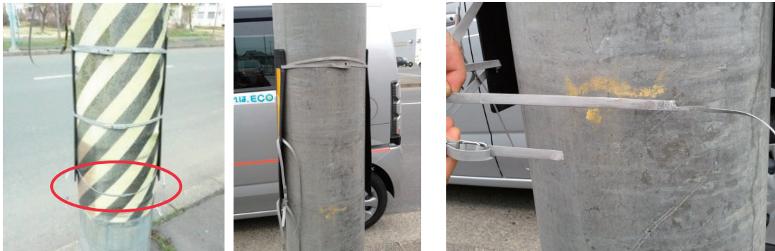
Fig. 1. Breakage of vinyl bands securing utility pole signboards.
