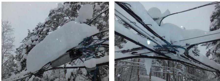
Fig. 2. Snow accretion on overhead equipment.
