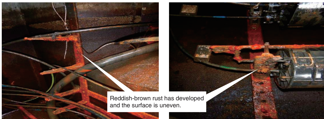
Fig. 7. Appearance of metal corrosion on fixtures inside a maintenance hole.
